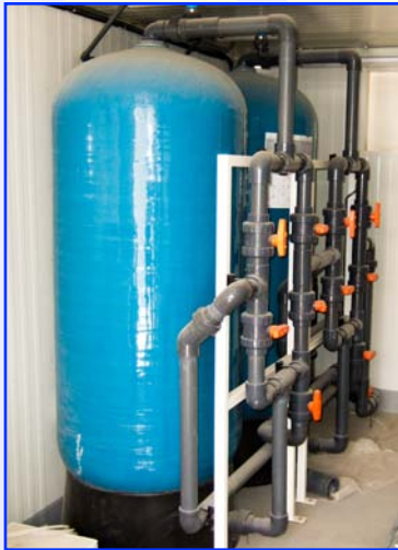
Tertiary Treatment Pressure Sand Filters. Auto or manual backwash.
