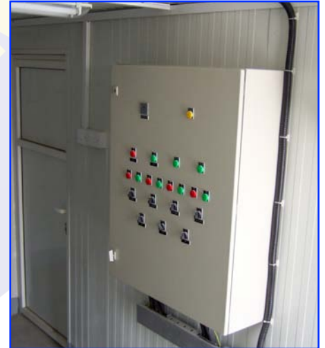
Standard switchgear control panel and motor PLC
