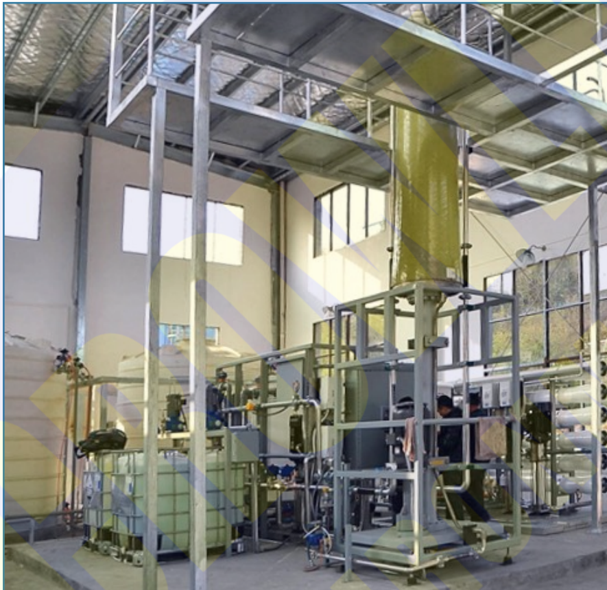
Typical Example of a Three Stage Membrane Plant Processing 65 tones per day slurry.
