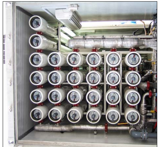
Typically arrangement of membrane housings for a containerised RO with a production capacity of 450 cubic metres per day. This particular plant include spare membranes which could be brought into use by the operator.
