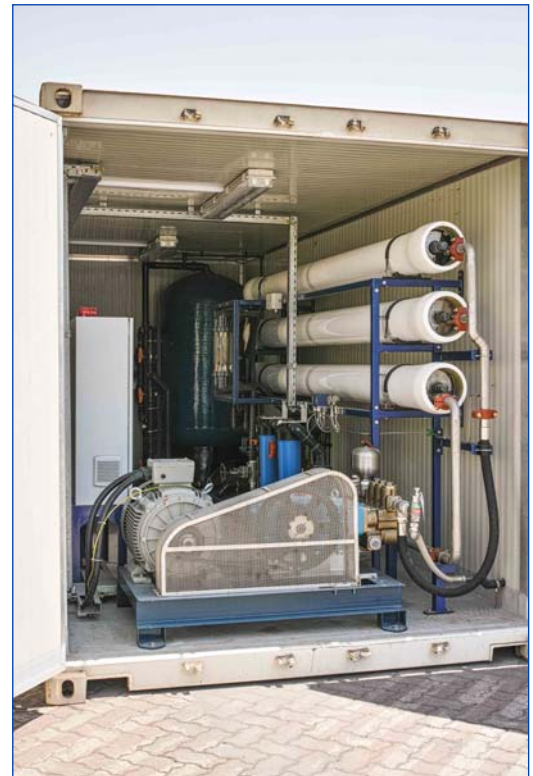
RO containerised Sea Water Reverse Osmosis package plant with a production capacity of 100 cubic metres per day
