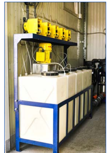
Chemical dosing system. Diaphragm doing pumps for pre and post chlorination, de-chlorination and pH adjustment.
